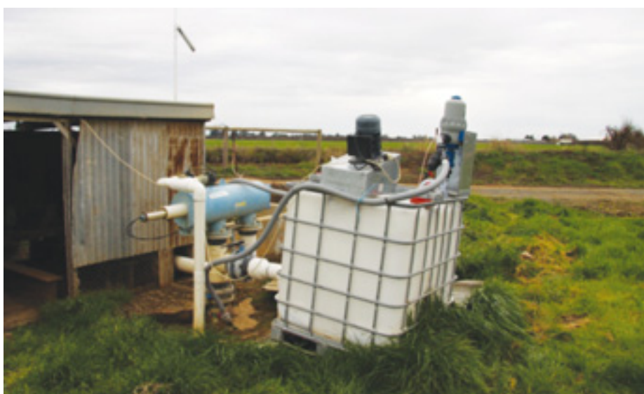
Combined unit with 1000L stock tank, electric agitator and Mixrite TF10 injection unit installed at a central farm point.
